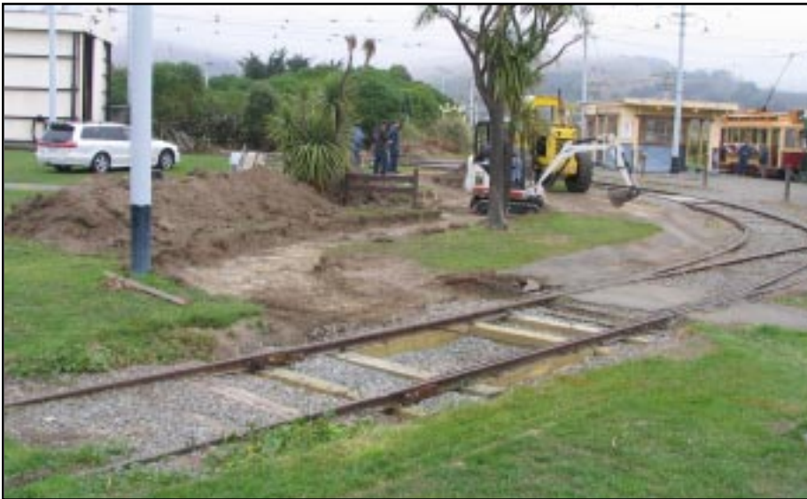
Tar seal is being removed to allow replacement of sleepers under the Gisborne point. The realignment will make trailer shunting safer and easier, and track maintenance easier.
